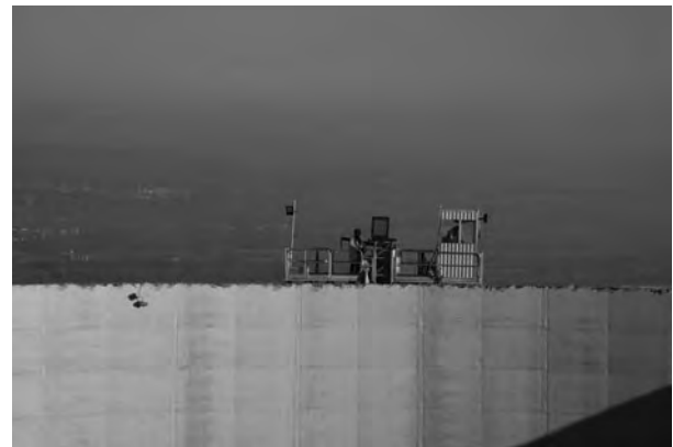
Figure 2: Conventional operation of the excavator with a handheld remote control from a platform on top of the cooling tower.
